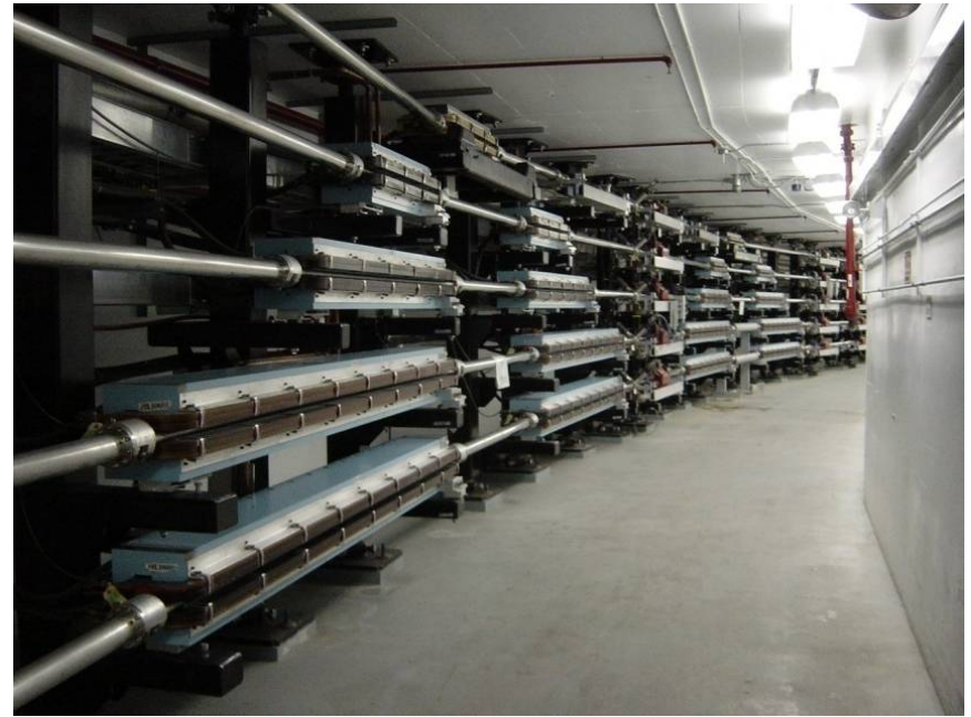
East side recirculation Arcs (5)
